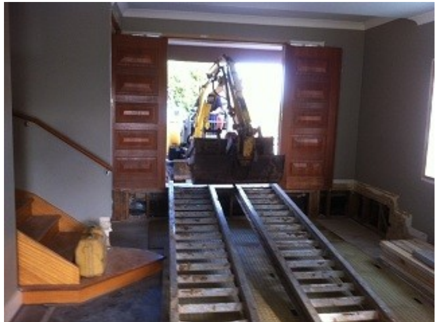
The ramps in place ready to transport the excavator into the backyard
